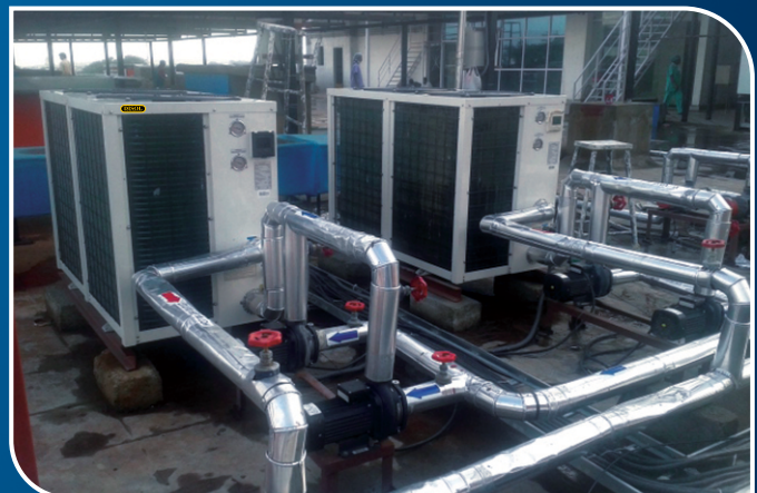
10,000 Ltrs. Capacity Hybrid System Installed : Sparsh Super Speciality Hospital, Bangalore
